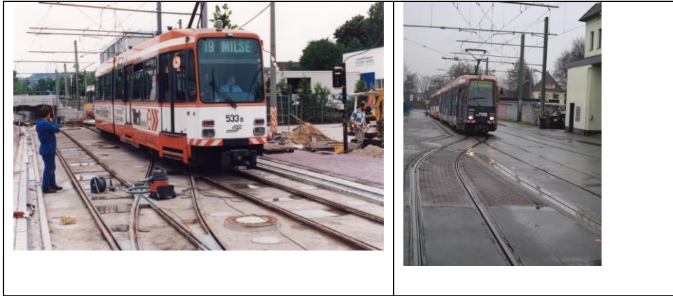
Figure: 4 Tram passing over a floating slab left: during construction and right: today
